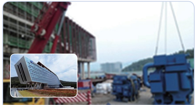
Korea Gas Corporation Daegu Office 2AB 1,300usRT(4,571kW)
