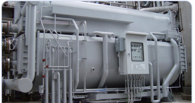
Lotte Petro Chemical Factory Explosion-Proof Steam Abs. Chiller, HWAR-L 7,800usRT(27,425kW)
