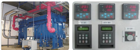
▲ 1st Generation Single Effect Double Lift Hot Water Driven Absorption Chiller
