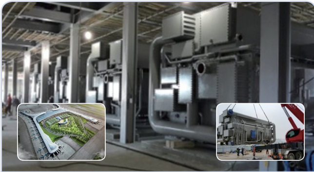
Incheon Interational Airport 2AB 8 sets 8,000usRT(28,128kW)
