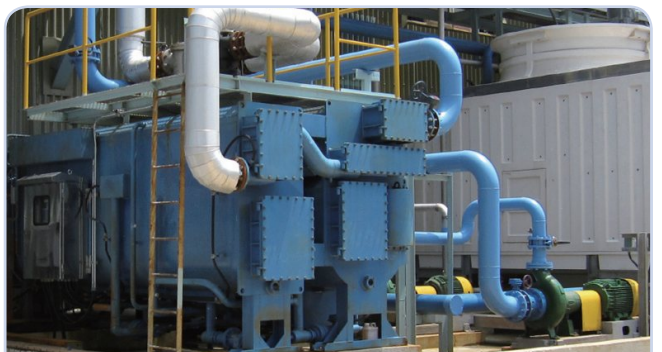
Youngpoong Seokpo Refinery 2AA 240usRT(844kW)
