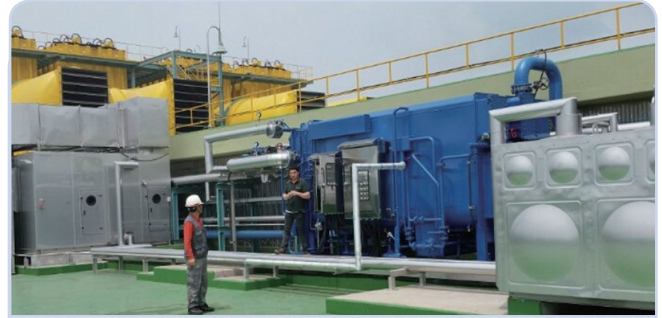
Korea Zinc. 2AA 210usRT(738kW), Air Handling Units Chilled Water Tank, Air Duct
